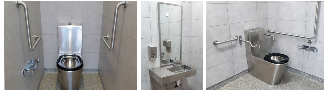
(L-R): Top - A view of the new Elgar Park sports pavilion, views of Britex Stainless Steel Accessible Bellagio Basin, Britex Stainless Steel Ambulant Toilet Suite, Britex Stainless Steel Accessible Bellagio Basin, Soap Dispenser and Framed Mirror, Britex Stainless Steel Accessible Toilet Suite.
